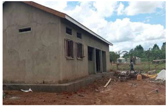
In Lamwo, the construction of a Police post and a female prisons ward are ongoing. Left is the female ward with works ongoing.
