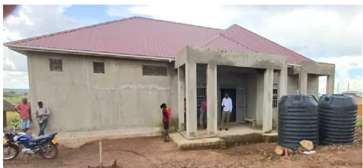
At Ofua IV in Rhino camp (Madi-Okollo), the project is at 80% level of completion. The plumbing works are ongoing. Remaining with plastering, shuttering and finishes.
