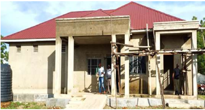
Kato - Imvepi refugee camp (Terego), the roofing of the structure has been completed. At finishes level. Works ongoing
