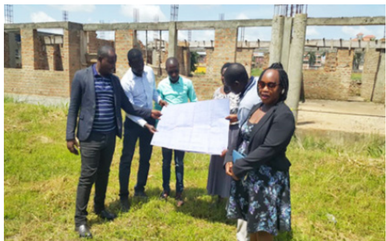
The UHRC Officers and an Engineer from JLOS handing over the architectural building plan to the Contractor at the site
