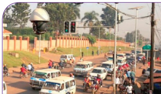
CCTV camera installed at a junction for traffic monitoring, incident management, and public safety.
